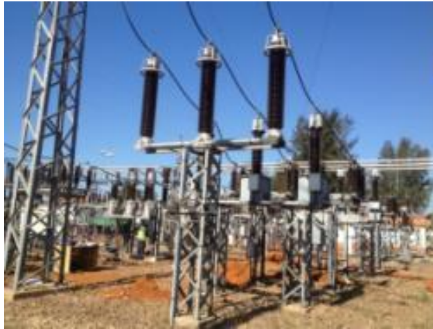
Improvement of Electricity Distribution Network - Maputo City
