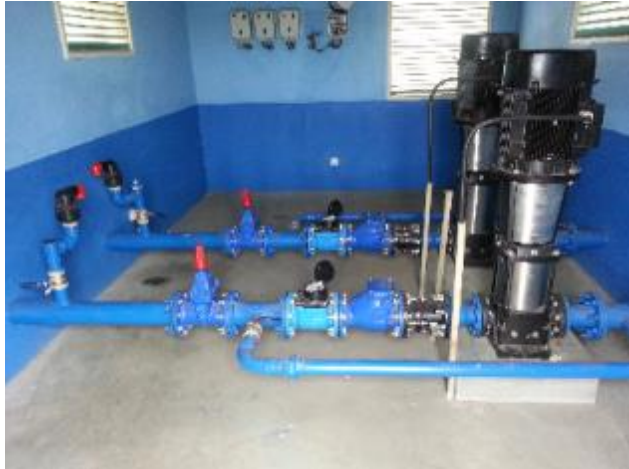
Pumping Station for Water Distribution System of Caia Village
