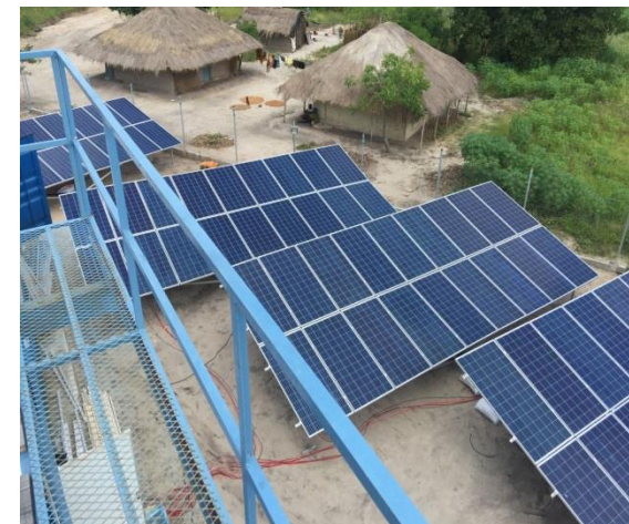
Mini Solar Power system for Health Centers Cabo Delgado
