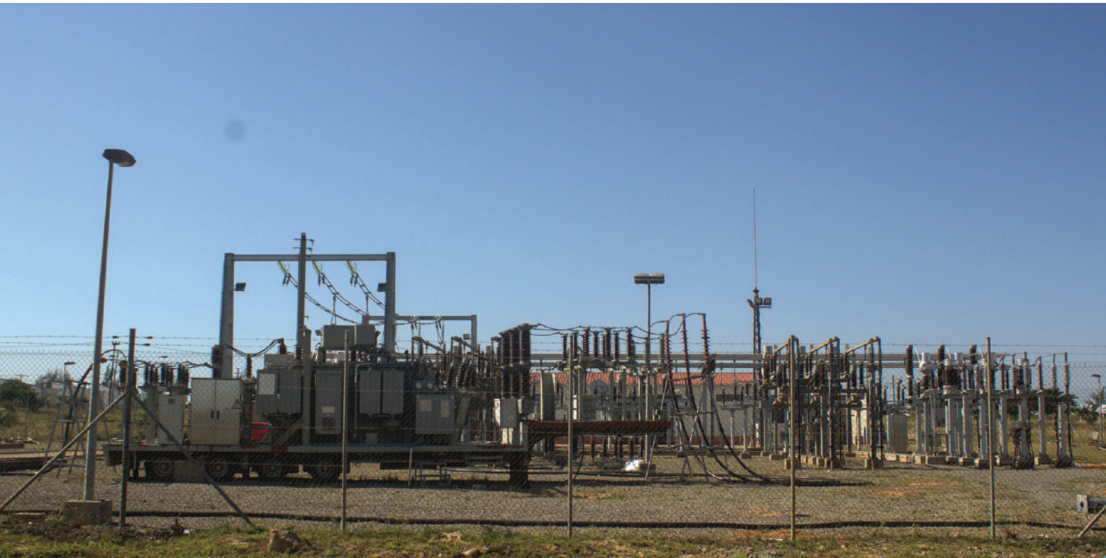
Zimpeto Power Substation – Maputo
