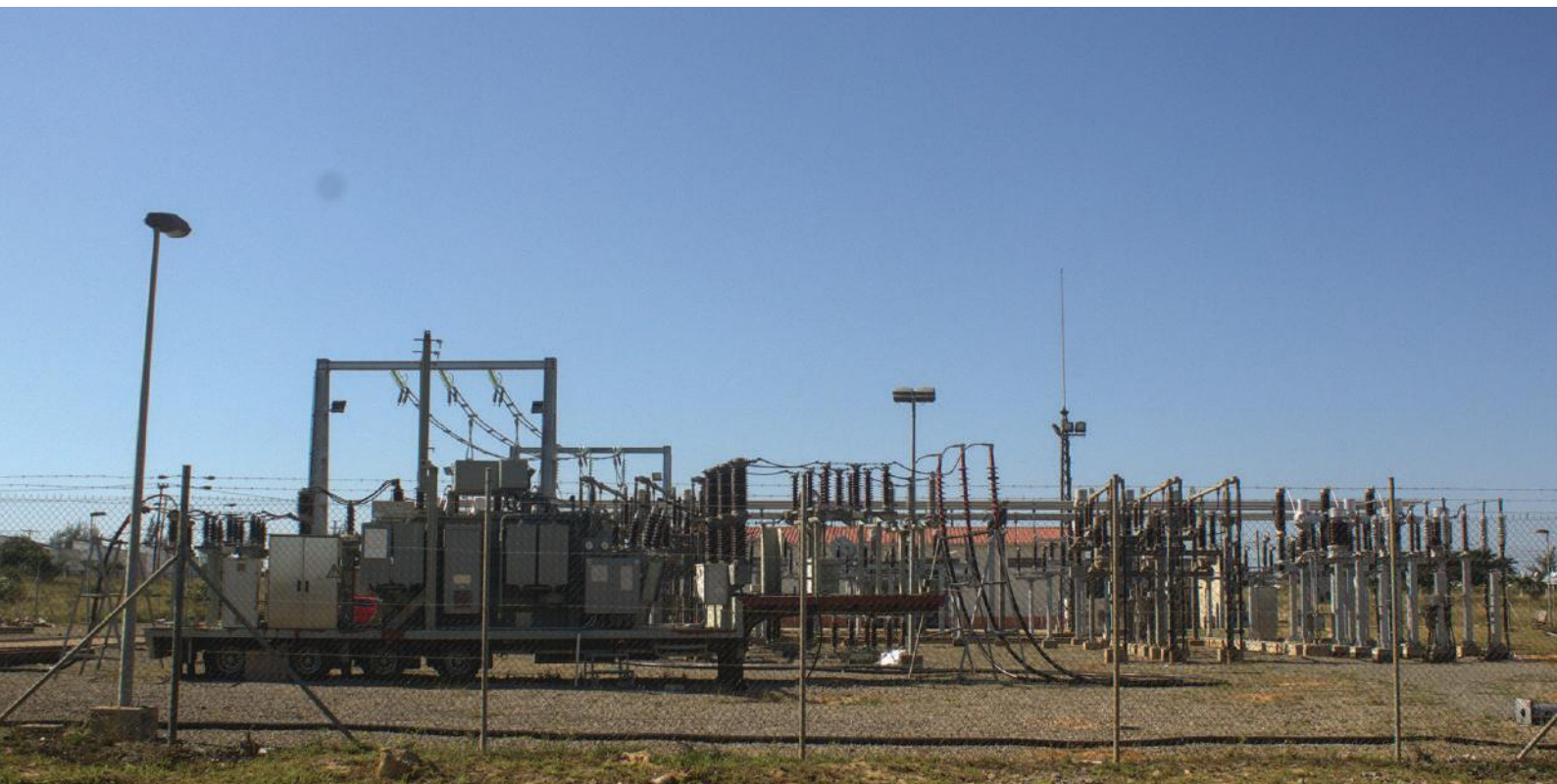
Zimpeto Power Substation – Maputo
